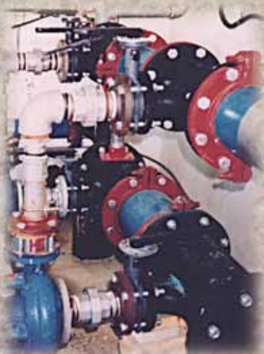
Series 900 Flange Adapters in a high pressure water pumping station.
