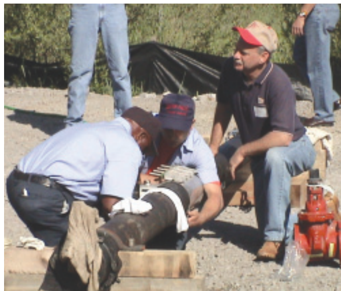
Don Fierstos, District Manager for Pennsylvania, New Jersey and Western New York, oversees the installation of a Ford FAST tapping sleeve during a live tap demonstration at a Pennsylvania Rural Water training session in Natrona Heights, Pennsylvania.
